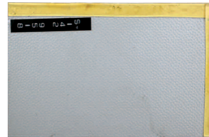
Figure 15. Colorcoat HPS200® with Galvalloy® metallic coating – 10 years exposure at Bohus Malmon, Sweden.
